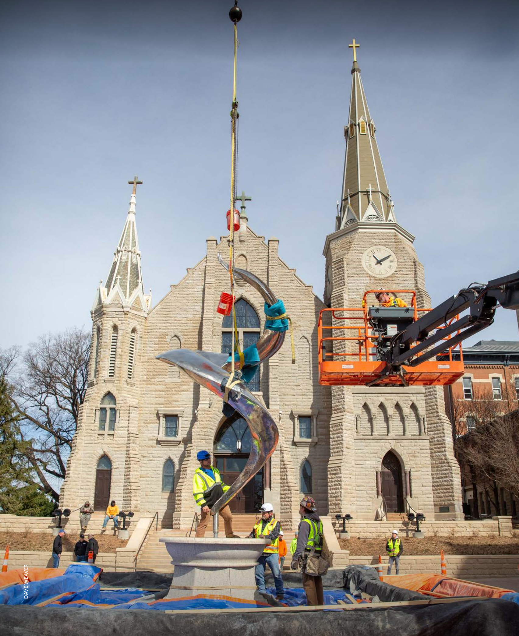
© In early March, the steel flame outside of St. John's Church was reinstalled after undergoing refurbishing and polishing during the renovation of the fountain and update to the St. John's plaza. The sculpture, "Eternal Flame," was originally installed in 1993, funded by a gift from John Micek, BS'50, and Anna Lou Micek, BA'75.
